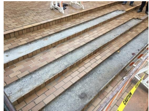
Figure 5: Deteriorated steps at Macmillan Building
